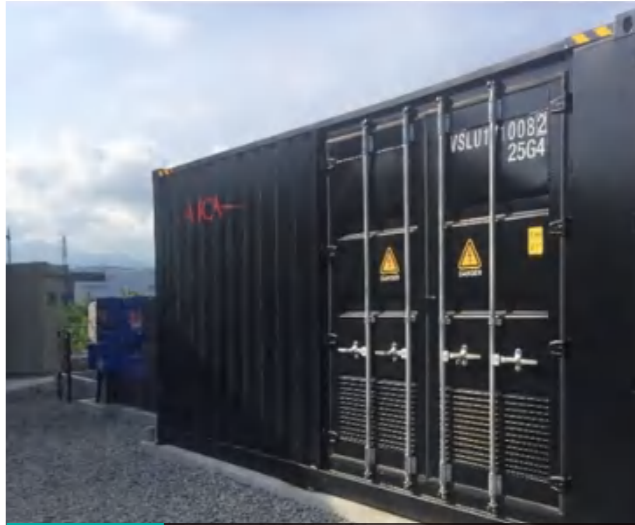
SENDAI JAPAN 540KWH/250KW Micro-grid Self-consumption Commercial ESS PV+DG+BESS
