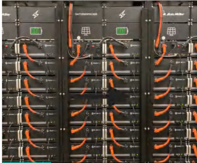
GERMANY 213KWH/100KW Peak Shaving Arbitrage Grid service ESS Grid+ESS
