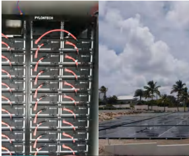
URUGUAY SOUTH AMERICA 750KWH/500KW Micro-grid Self-consumption ESS PV+BESS
