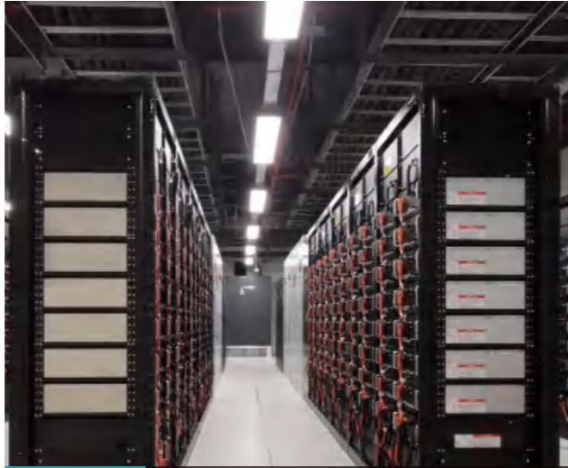
SHANGHAI CHINA 2MWH/1MW IDC UPS Back Up Grid+BESS
