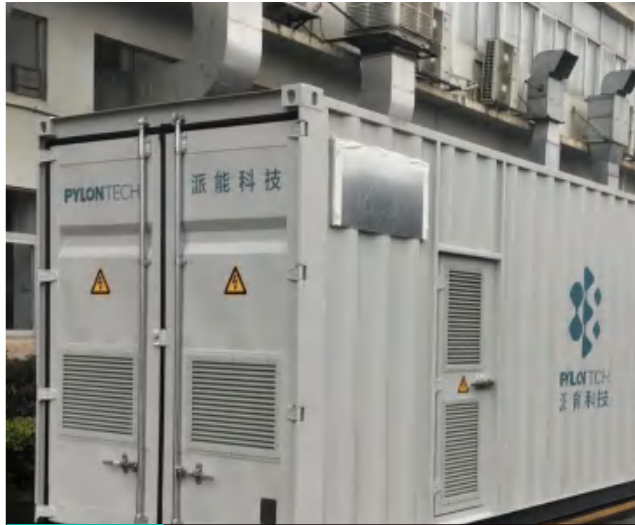
SOUTH EAST ASIA 624KWH/50KW Micro-grid Self-consumption ESS PV+DG+BESS
