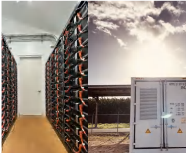
U.S.A. 2.MWH/1MW Self-consumption/Back-up Commercial ESS PV+Grid+BESS
